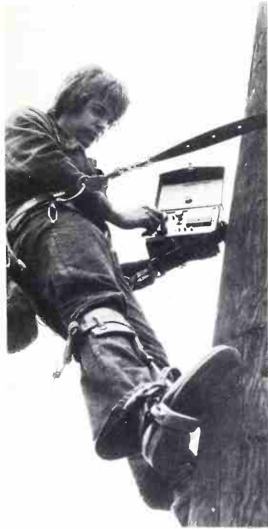
Rapid location and remedy of malfunctions in major components will be a necessity in the future.
